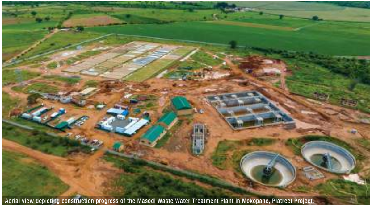
Aerial view depicting construction progress of the Masodi Waste Water Treatment Plant in Mokopane, Platreef Project.
